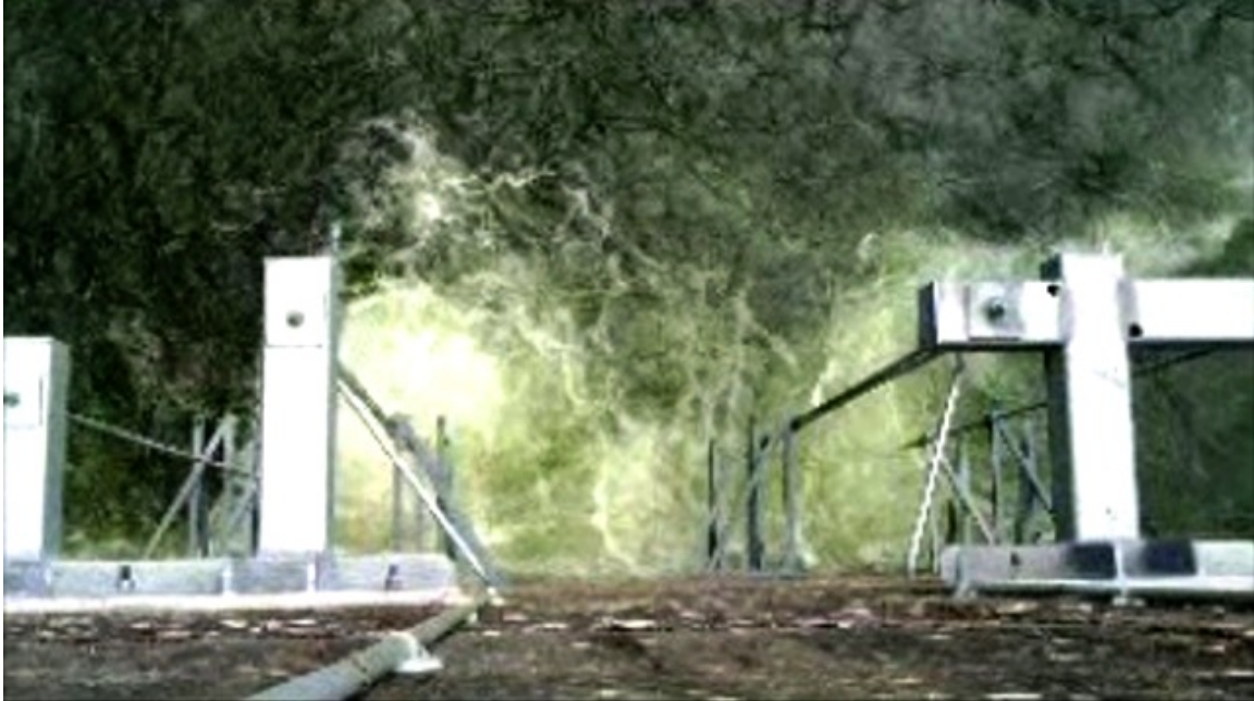
Figure 1. Boil of water and air emanating from the Lamprey Flume System (LFS). This boil appears when the valve controlling water supply to the LFS is set at approximately 70% open or greater. The Corps is concerned that the boil may indicate either an open access hatch or physical damage to the flume, either of which would pose a fish passage risk. The purpose of the ROV inspection was to verify that this is not the case.
